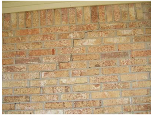
The brick veneer crack needs to be repaired.
