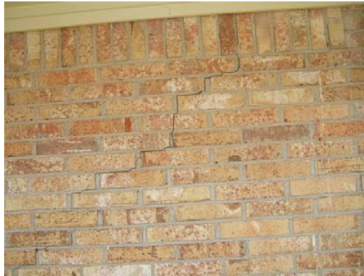
The brick veneer crack needs to be repaired.
